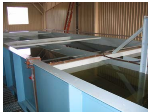
Snake Creek Water Plant Treatment Unit
